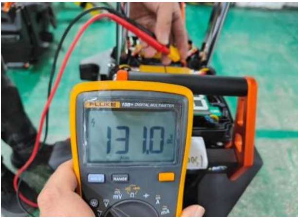
14 Full battery voltage check
