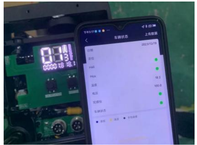
Battery voltage check By App:
